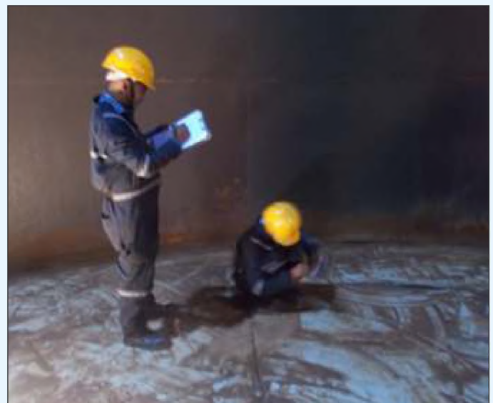
Photo 5: Manual Thickness survey of FWT 05 bottom plate
