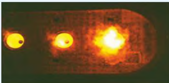
Figure 6: Improper Burner operation leading to flux maldistribution
