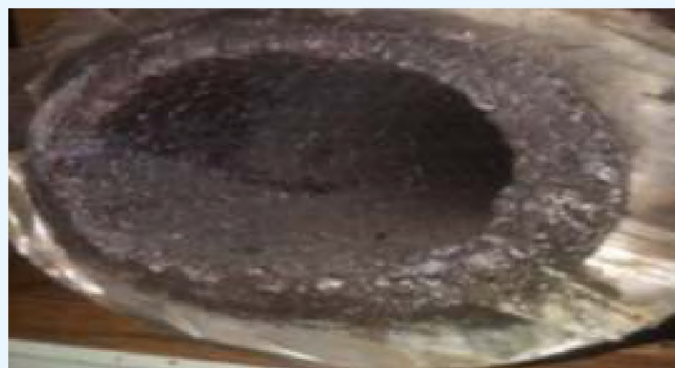
Figure 7: Accelerated fouling at reduced load
